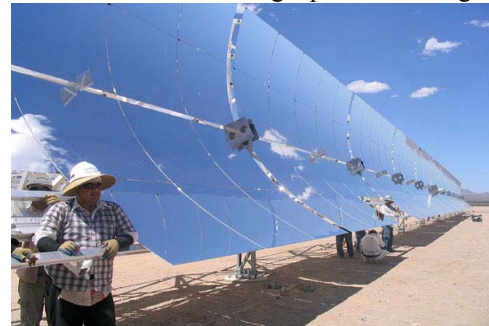
Fig. 7 Solar Power Plant
